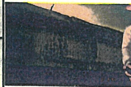
The Wooden Fender was Brocken cannot reduce the ship Force.
